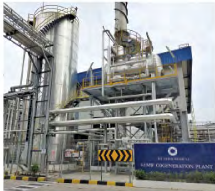
Our CoGeneration Plant in Johor
