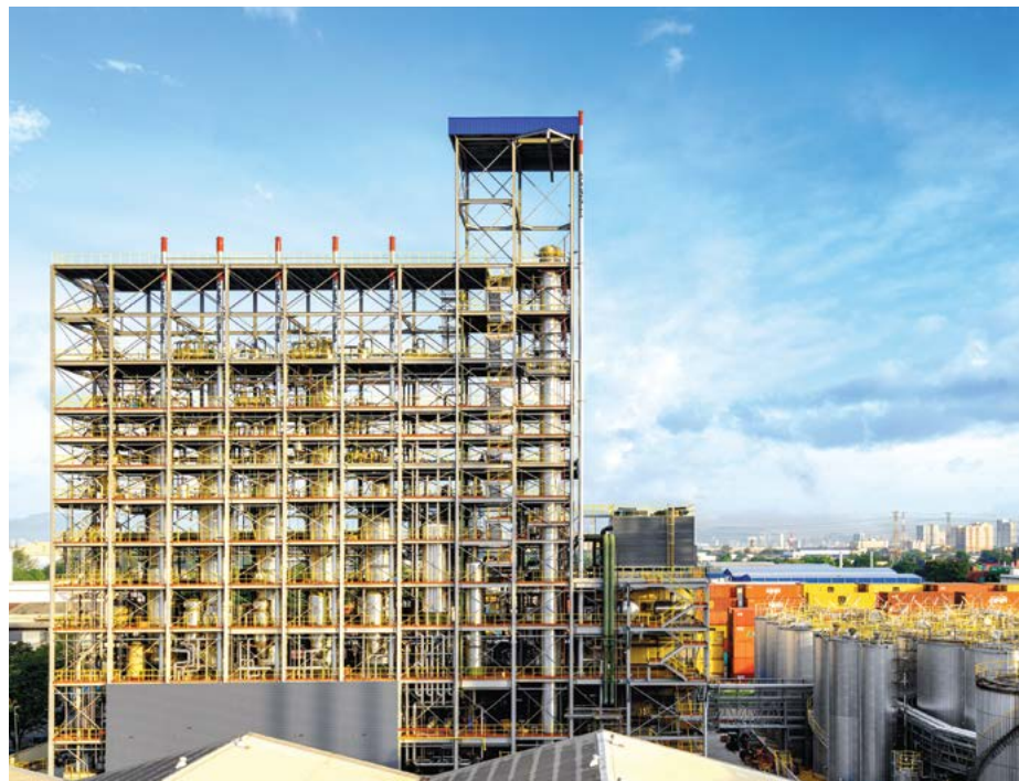
Our new oleochemical plant in Prai, Penang will increase the Group's oleochemical production capacity by about 14% to 890,000 MT/year.
