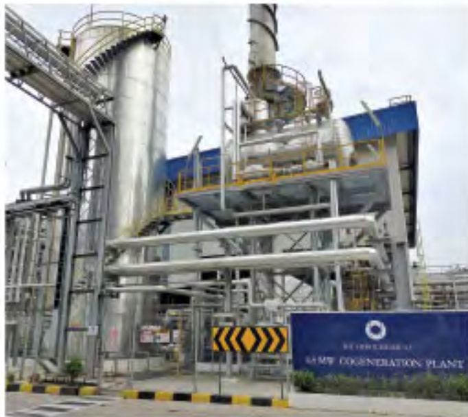
Our CoGeneration Plant in Johor
